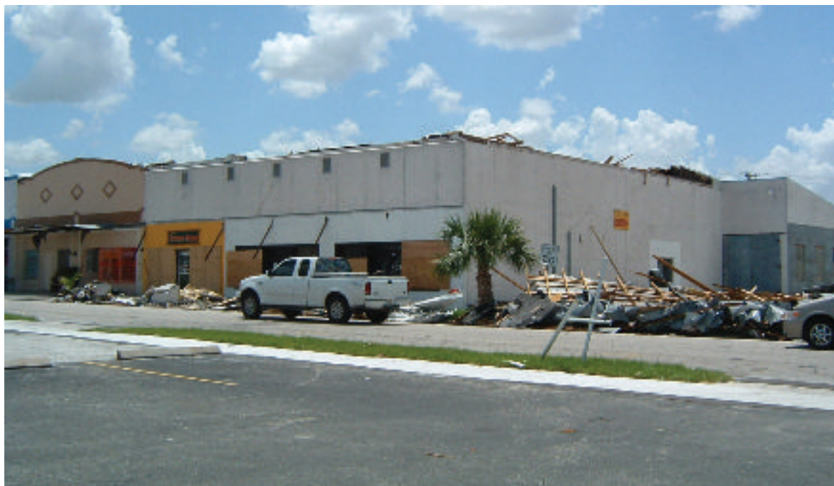
The Sarasota County History Center conducted a damage survey in Arcadia after Hurricane Charlie (shown above) and used this experience to develop steps in their Action Plan. SARASOTA COUNTY HISTORY CENTER
