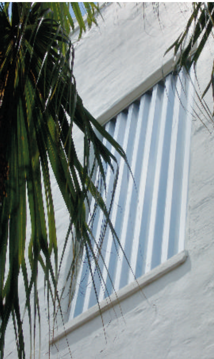
Protective panels for windows and doors, shown here on the Bonnet House, can help reduce the cost of insurance. BONNET HOUSE MUSEUM AND GARDENS
